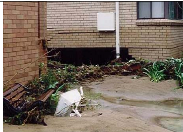
Fig. 30. Damage to brick building
